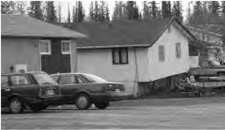
Figure 9: Houses near Fairbanks, Alaska use jacks for support as permafrost thawing causes uneven settling. Source: ©1999, Gary Braasch.
